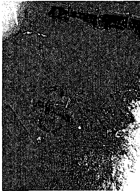
Popcorn ceiling debris
